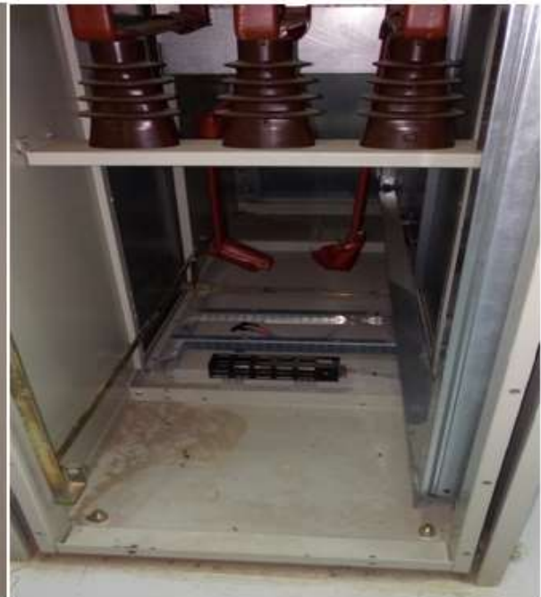
Figure: Space for installation of new VTs
