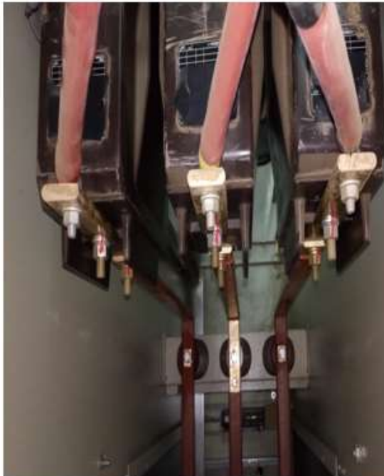
Figure: Existing CTs- to be replaced
