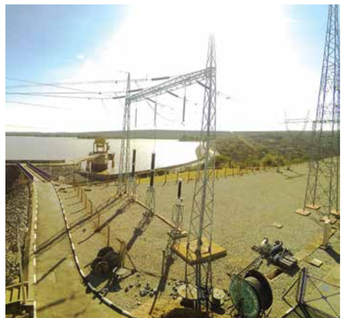
Kamburu Power Dam and transmission station at the Eastern Hydropower business area. Hydro is still a key component of the Company's generation mix.
